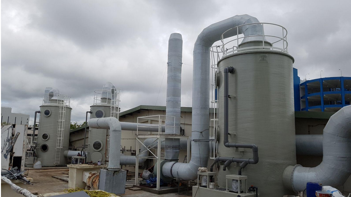
Acid and cyanide scrubbers at Cimelia
